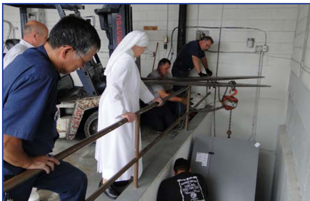
Director of Maintenance, Chito Rilloraza and Mother Marguerite watch as one of the new boilers is lowered into the basement.
